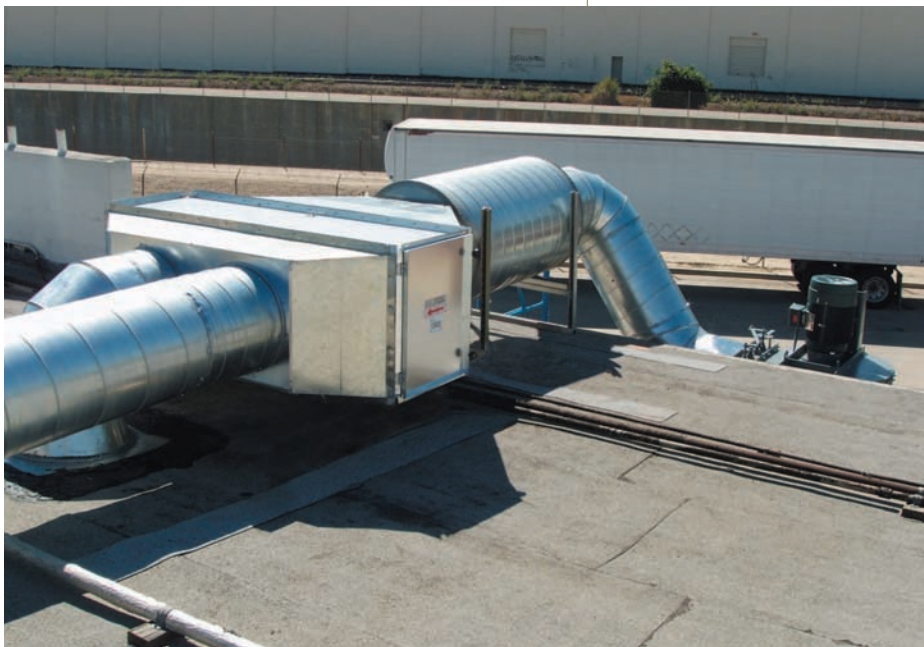
A view of exhaust duct from the SFC collector shows the system's in-line silencer and safety filter.
